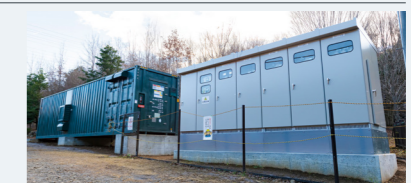
Storage batteries, power receiving and transforming facilities, distributed server facilities
